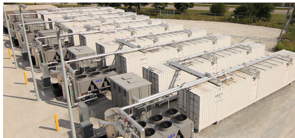
Utility Scale Batteries
