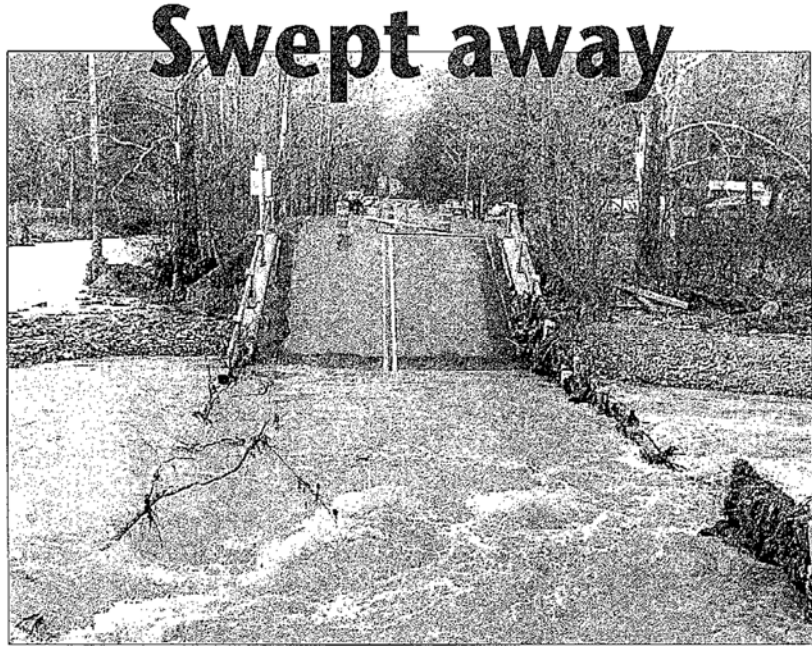
On Nov. 7, 1985, this was The Recorder's powerful front-page image of the bridge across Back Creek on U.S. 84, just east of Route 600, destroyed when high waters pulled the west end of the bridge from its supports shortly after noon on Monday, Nov. 4. It was captured by then news editor Winnie Richardson.
