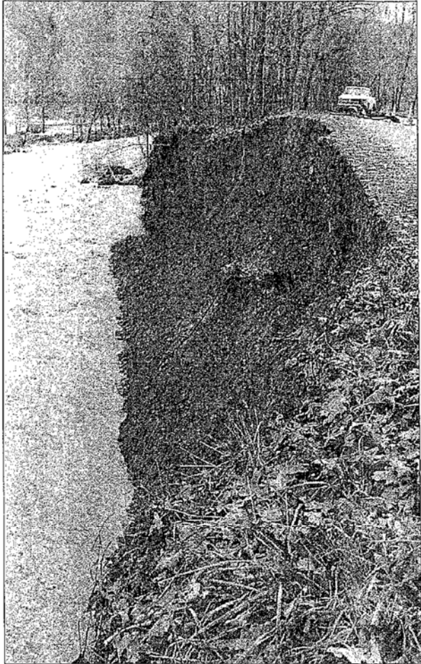
This section of Route 600 caved into Back Creek just north of the Virginia Power project property. The debris from the mud and rock slide blocked Lightner Bridge a short distance downstream, preventing workers from leaving the dam Monday afternoon. (Recorder file photo)
