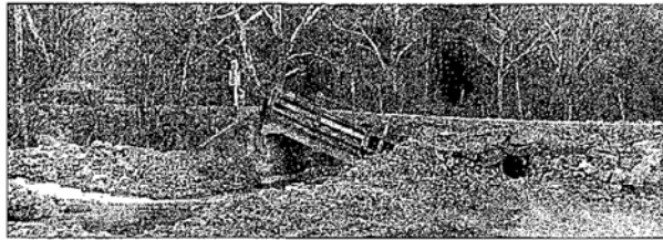
This small section of Route 84 near Route 600 and Back Creek caused questions and complaints from Monterey landowners for the state highway department at a Highland board of supervisors meeting following the flood. Residents were concerned repairs would not be handled quickly enough. (Recorder file photo)
