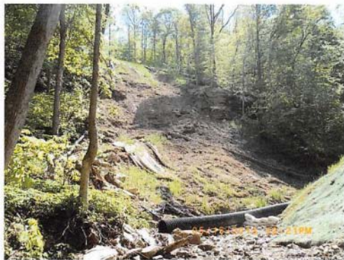
Photo 3: N 39° 52.3772' W 80° 41.1271' Bartletts Run. Flume pipe, sand bags and slip material in stream.
