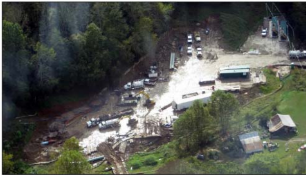
FIGURE VII(c) – Entry-side workspace for a comparatively small HDD operation for the Stonewall Gathering Pipeline in West Virginia. The pullback phase has been completed and the drilling rig has been removed. This operation involved a 1,000 foot boring to install a 36-inch pipeline under Interstate 79.
