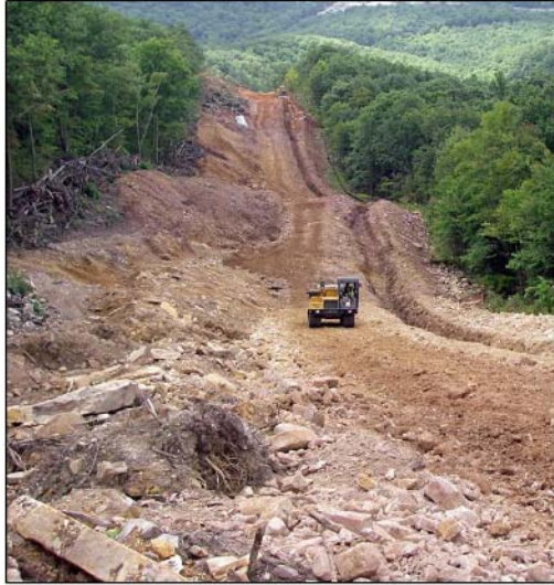
FIGURE VII(o) – A comparatively small 2014 pipeline replacement project in the Jefferson National Forest on Peters Mountain in Giles County, Virginia. A variance to the 500-foot open trench limit was requested for this project. Although slopes exceeded 40%, the DEQ approved the variance request, allowing a 2,000-foot open trench. No water interceptor diversions were installed during trenching. Following a rain event that occurred shortly before the above photo was taken, a Forest Service employee described having “never seen that much sediment move off site before.” A case-study report is posted at www.pipelineupdate.org/case-study-no-1/ . The Dominion Pipeline Monitoring Coalition conducted a study of open-trench variance requests for pipeline construction projects in Virginia. Fifteen variance requests were submitted between January 2011 and July 2014, and all were approved. The authorized open-trench lengths ranged between 500 feet and 15 miles, with an average length of 2.3 miles. Nothing was discovered in DEQ documents to indicate that an analysis was conducted to ensure that these variances would not cause illegal discharges and water quality degradation.
