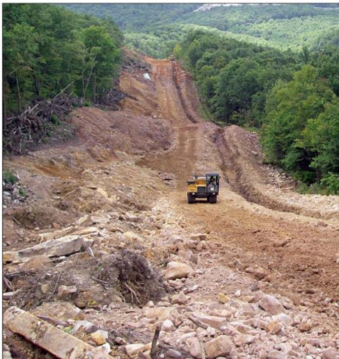
FIGURE 14 – A comparatively small 2014 pipeline replacement project in the Jefferson National Forest on Peters Mountain in Giles County, Virginia. A variance to the 500-foot open trench limit was requested for this project. Although slopes exceeded 40%, the DEQ approved the variance request, allowing a 2,000-foot open trench. No water interceptor diversions were installed during trenching. Following a rain event that occurred shortly before the above photo was taken, a Forest Service employee described having “never seen that much sediment move off site before.” A case study report is posted at www.pipelineupdate.org/case-study-no-1/ . The Dominion Pipeline Monitoring Coalition has conducted a study of open-trench variance requests for pipeline construction projects in Virginia. Fifteen variance requests were submitted between January 2011 and July 2014, and all were approved. The authorized open-trench lengths ranged between 800 feet and 15 miles, with an average length of 2.3 miles.
