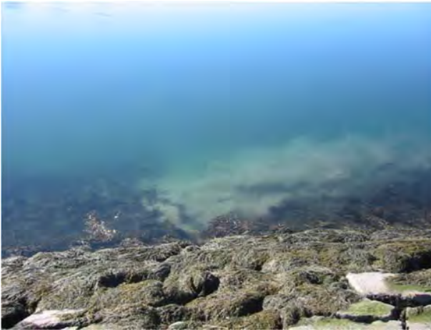
Figure 3: Inadvertent drilling fluid return in waterway
