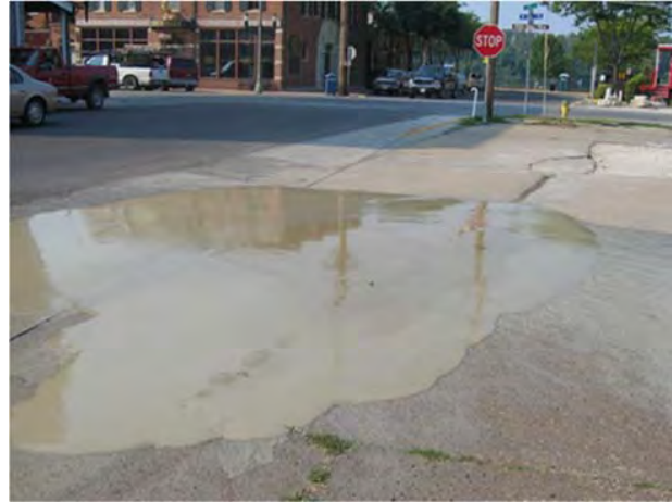
Figure 4: Inadvertent drilling fluid return surfacing through cracks in pavement
