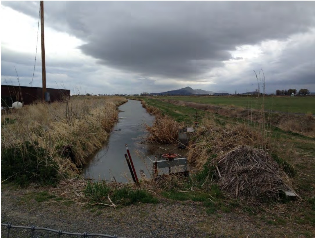
Crossing 21, D-3-A Lateral looking southeast. Image was taken approximately 650-ft northwest of the proposed crossing location.
