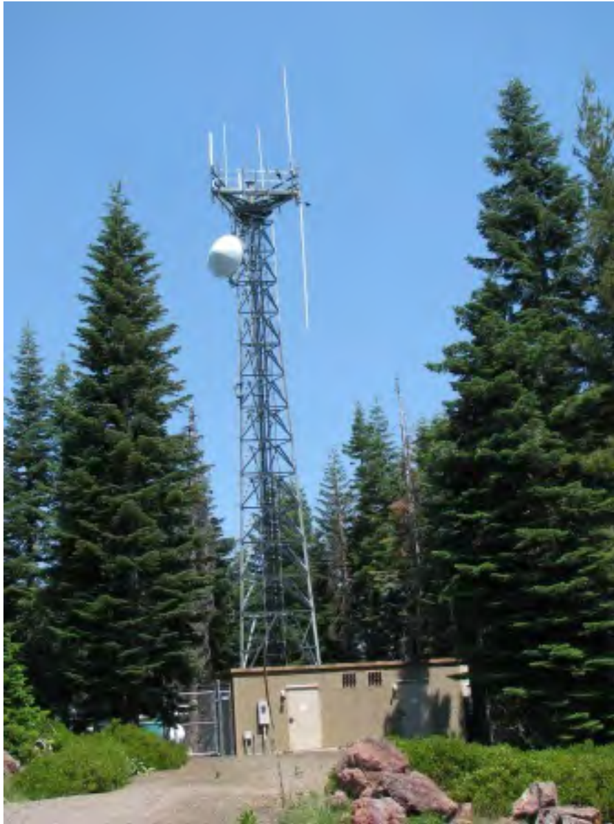
Facility 2 – Medford Cellular (ATT)
