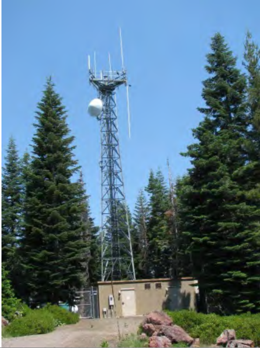
Facility 2 – Medford Cellular (ATT)
