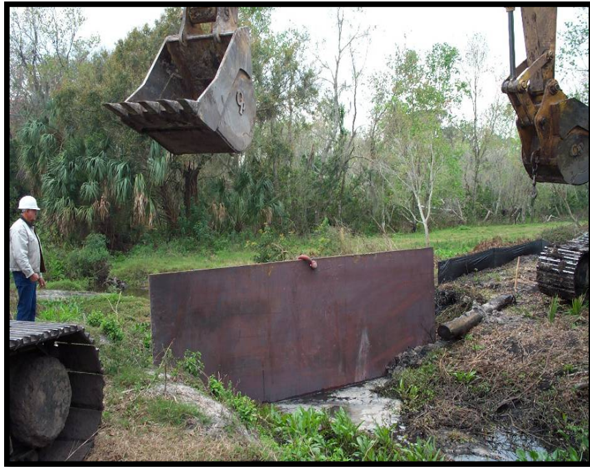
Figure 1-3 Installation of a Dam in a Dry Open-cut Crossing of a Small Channel
