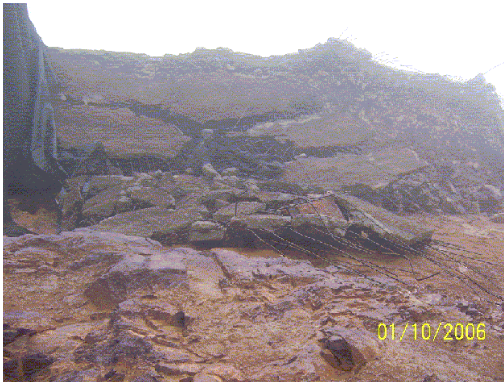
Figure 2.4 - View of bedrock immediately below failed embankment section. Note weathered clay in lower portions of the exposure.
