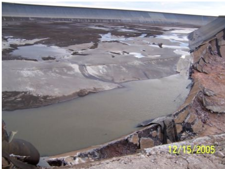
Figure 2.10 - Breached area. Note “fish pond” area immediately upstream of the breach. This area was over-excavated during original construction due to poor foundation conditions.
