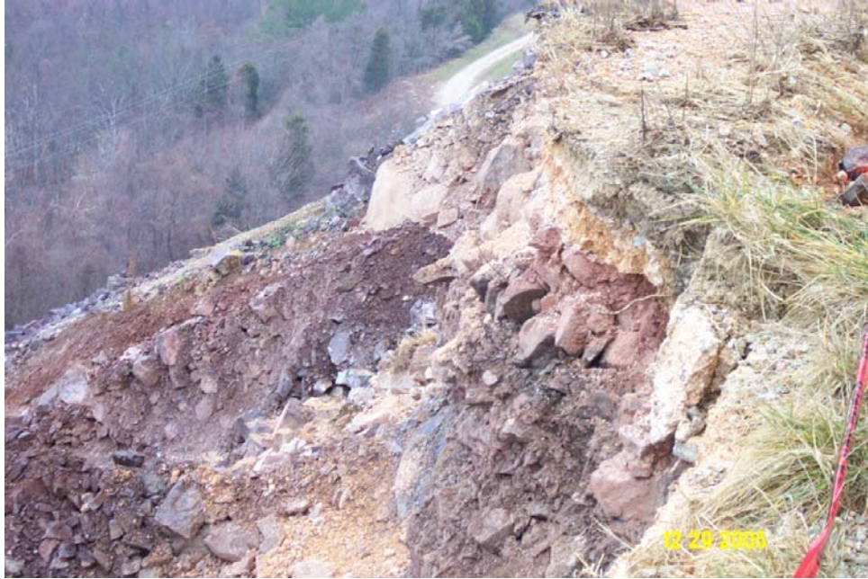
Figure 4.5 - Panels 48 and 49 Scarp near toe of parapet wall footing
