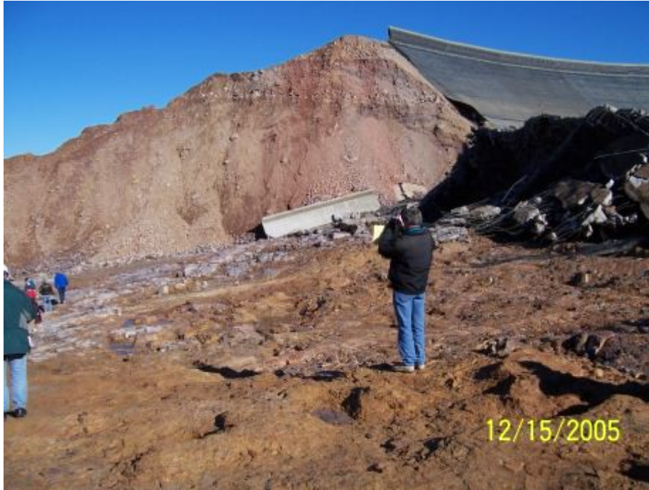
Figure 9.2 - Area of weathered rhyolite, which is in-line with the “fish pond” depression in the reservoir (background).
