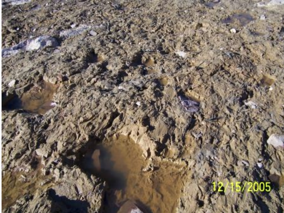
Figure 2.7 - Grooves cut into an area of clay-seam foundation by the floodwaters. This area is located immediately downstream and in the center of the breach.
