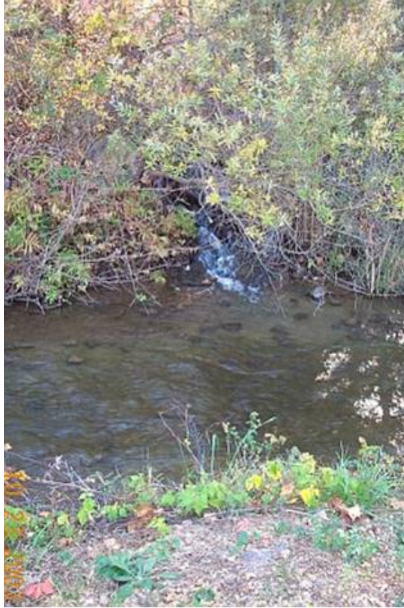
Figure 3.7 - Concentrated Seep Before liner installation (2003 FERC Operation Inspection Report)
