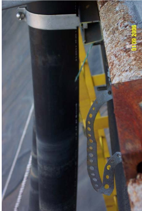
Figure 5.6 - High Water marks on HDPE Tubes
