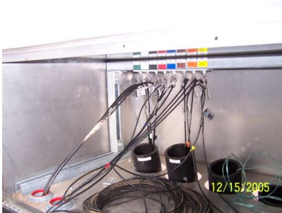
Figure 5.2 - Cabinet containing the Druck pressure transducer and Warrick conductivity sensor wiring
