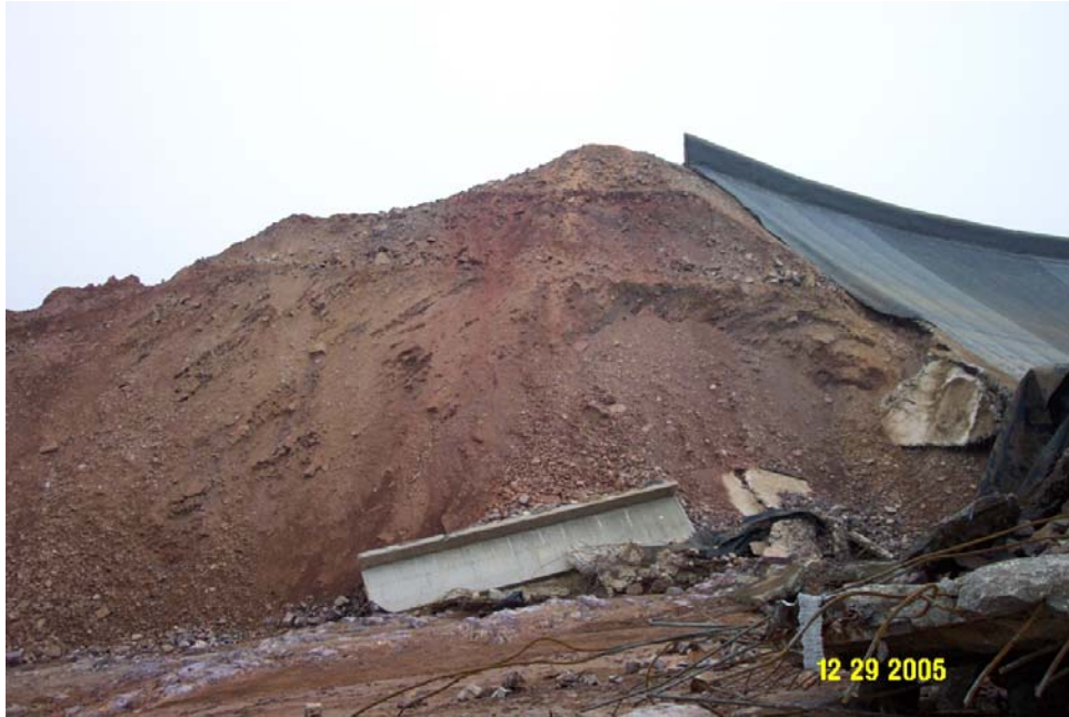
Figure 4.12 - Right side of breach Note layering of embankment
