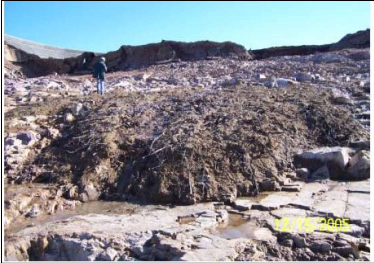
Eroded foundation, note rock jointing and overlying clay materials
